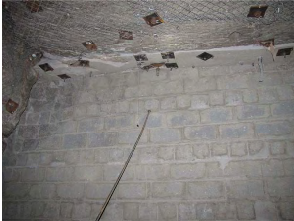
Figure 5. Surface spalling at the top corner of the explosion wall in the intake drift of Panel 1 during February 2012.
