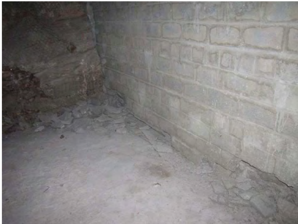
Figure 4. Surface spalling at the base of the explosion wall in the intake drift of Panel 1 during February 2012
